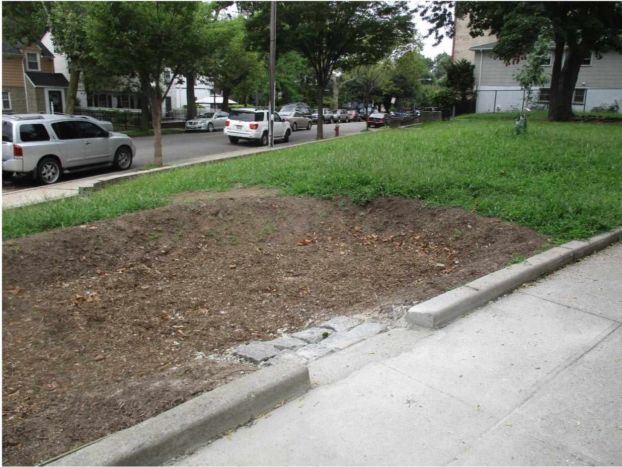
Construction Day 4: August 10, 2016 – Jersey City DPW completed the curb cut and added additional mulch to the rain garden.
