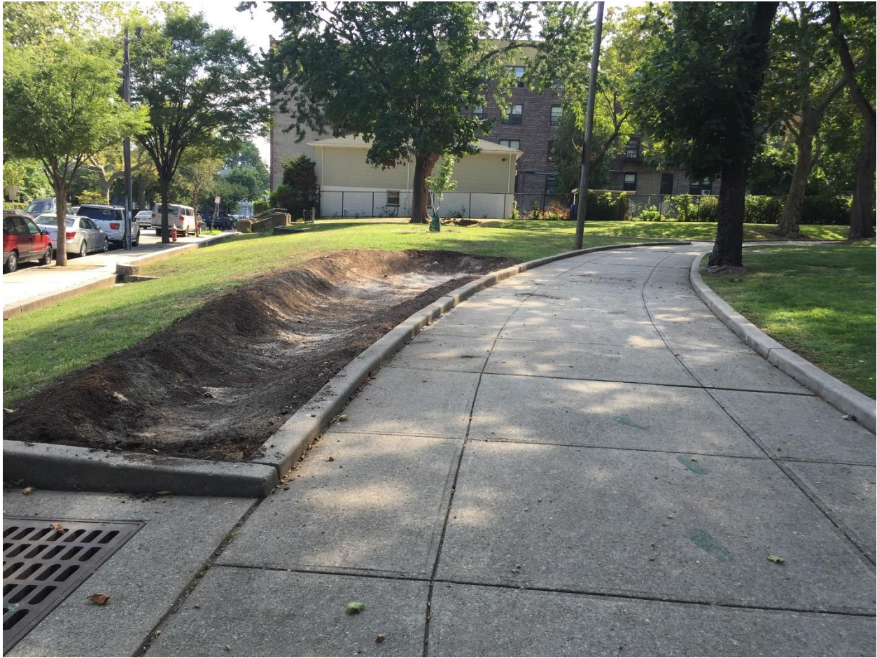
Construction Day 3: July 21, 2016 – The RCE Water Resources Program added additional sand mixture to the base of the rain garden.
