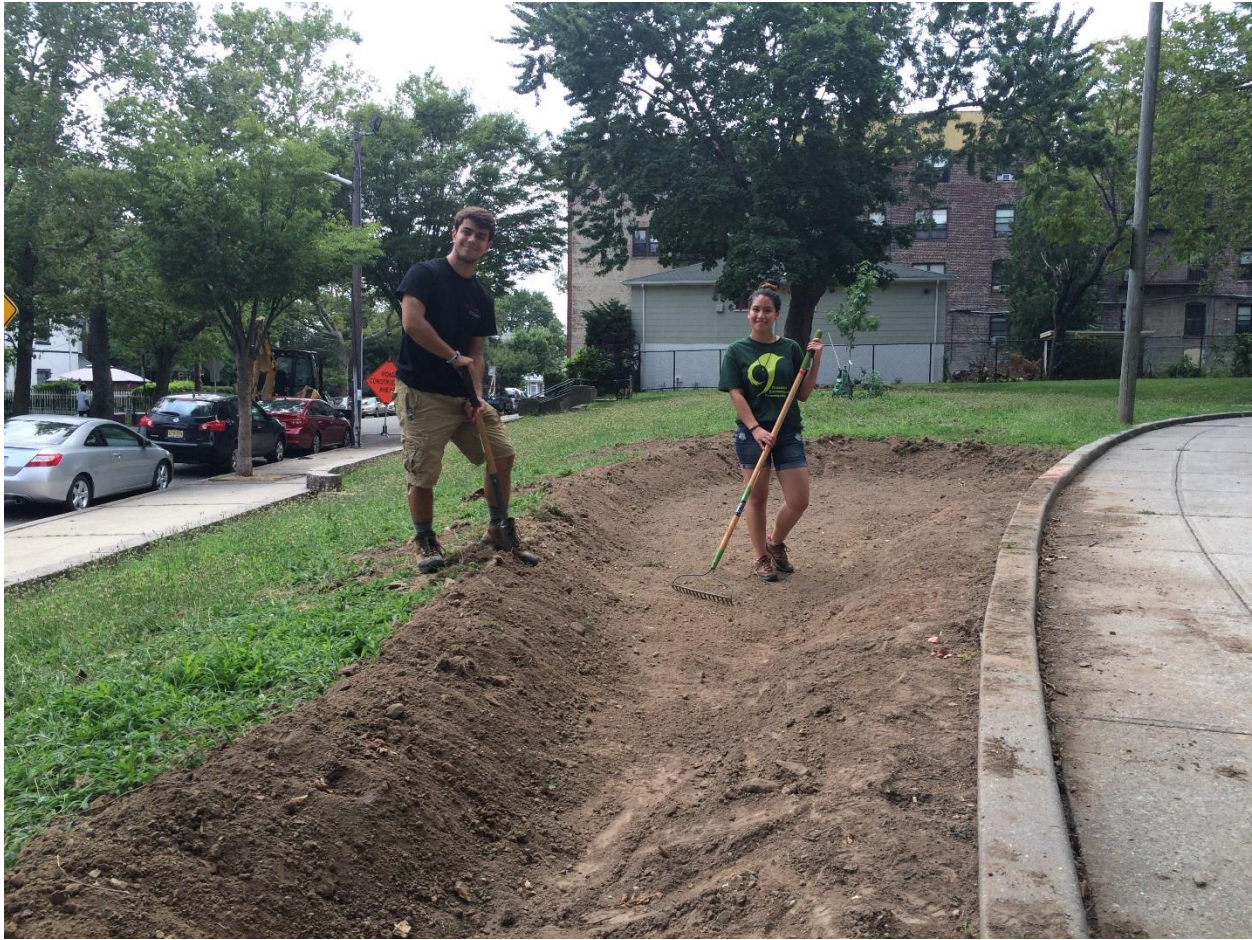
Construction Day 1: July 13, 2016 – Ms. Balladares, the RCE Water Resources Program, and the Jersey City DPW excavated the demonstration rain garden.
